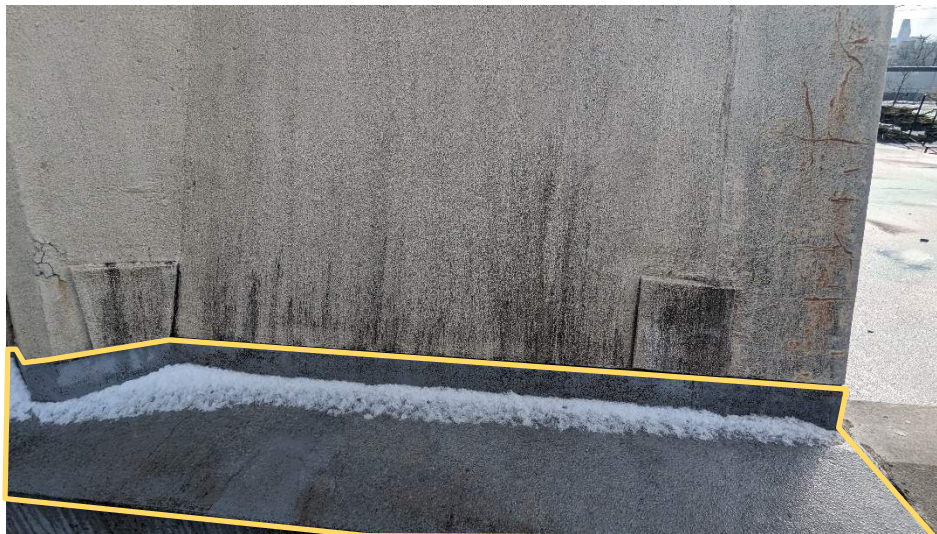
Photo 7: Projection de la dalle structurale - condition saine
