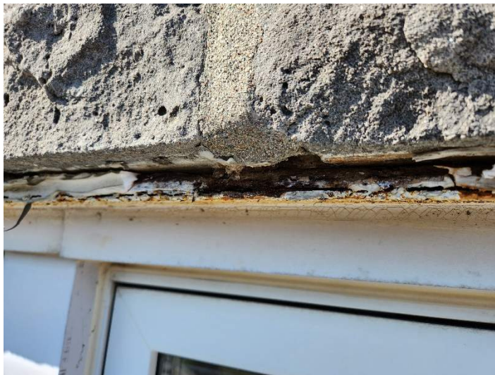
Photo 14: Corrosion des linteaux (source DMA)
