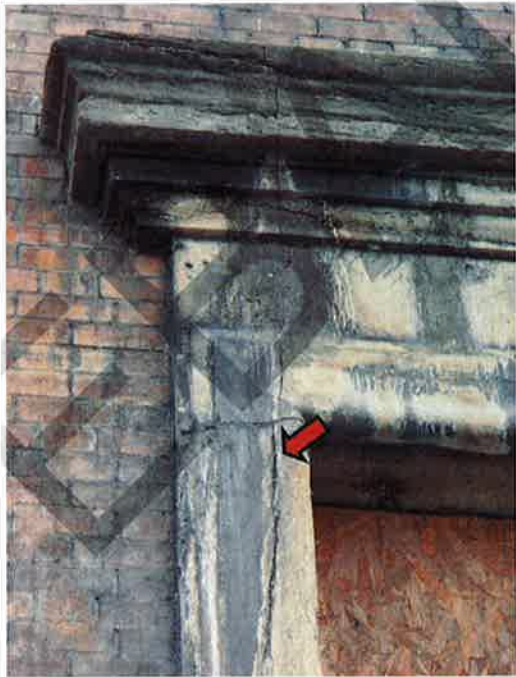
Photograph No. 14: Vertical crack in dripstone over window opening (east façade)
