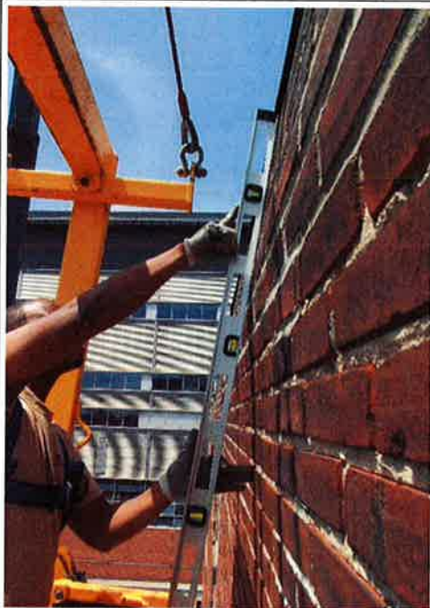
Photograph No. 20: Severe bowing/lateral deflection of the brick masonry cladding (west façade) (CRITICAL CONDITION)
