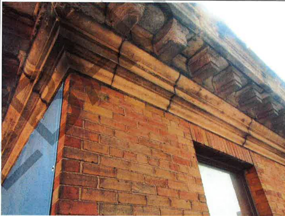
Photograph No. 56 : Building 1162 : Erosion of string course stone (west elevation)
