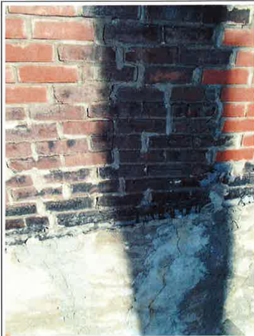
Photograph No. 28: Fissured mortar joints and cracked cementitious parging (south façade)
