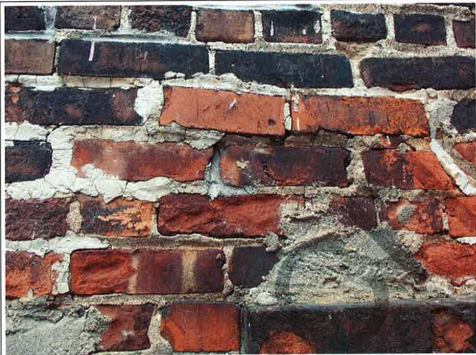
Photograph No. 81 : Building 1180 : Typically poorly repointed mortar jointing (north elevation – roof level)
