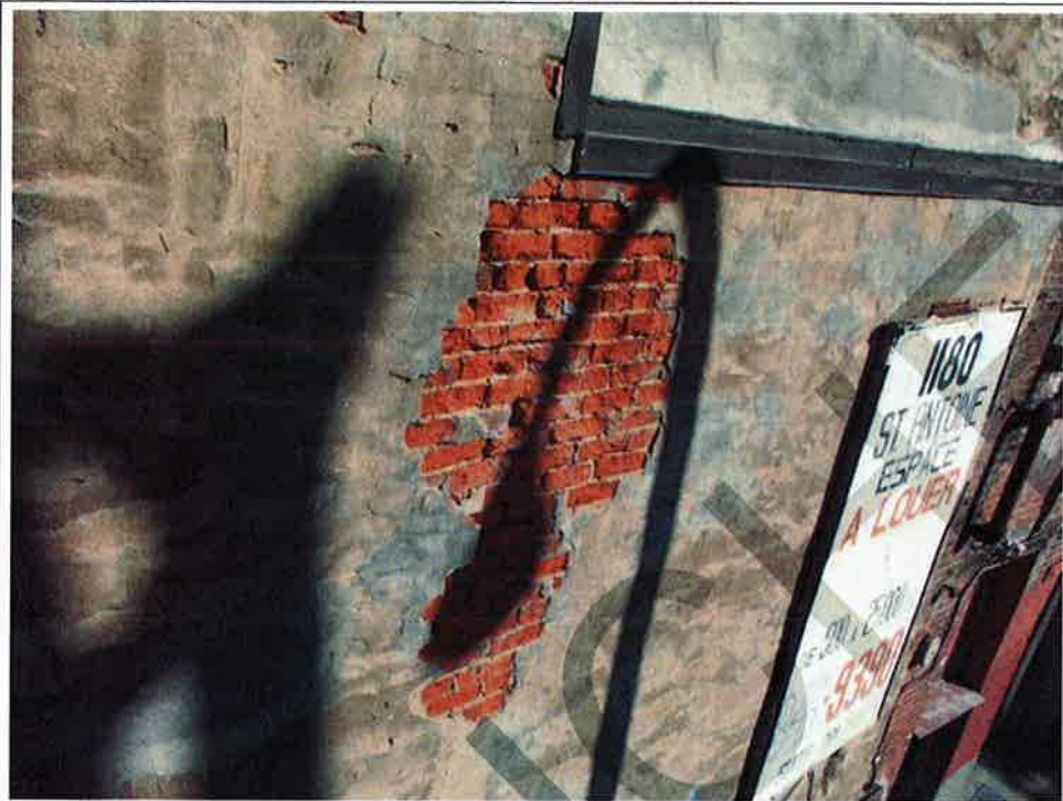
Photograph No. 35: Typical deteriorated and cracked cementitious parging, exposing spalled brick units (south façade)
