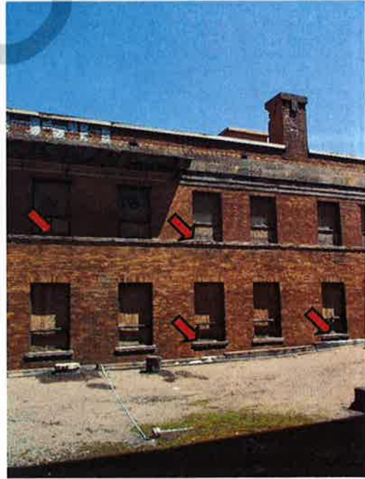
Photograph No. 15: Widespread erosion and spalling of stone window sills and string courses (west façade)
