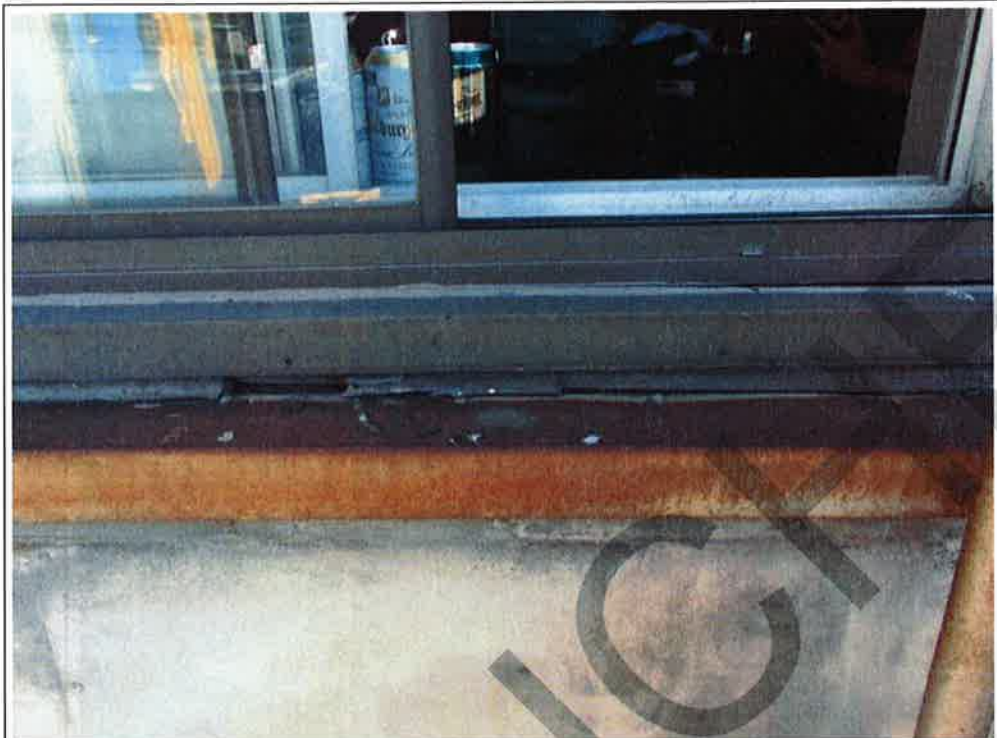
Photograph No. 37: Typical sign of heavily deteriorated or missing caulking of joints surrounding window frame (west façade)
