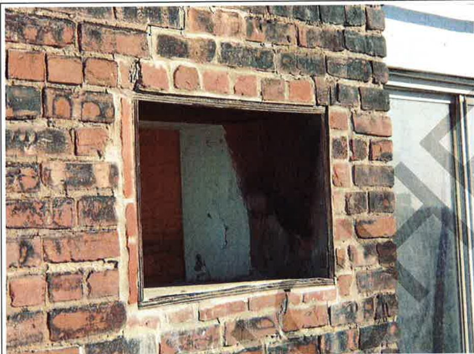
Photograph No. 85 : Building 1180: Typical inadequate waterproofing at opening through wall (south elevation)
