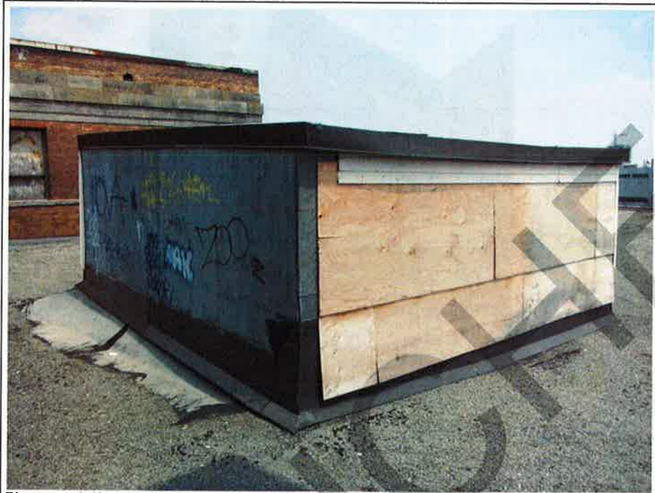
Photograph No. 79 : Building 1180: Typical patching of exterior walls by penthouse (note the vinyl siding, sheet metal and plywood) (roof level)
