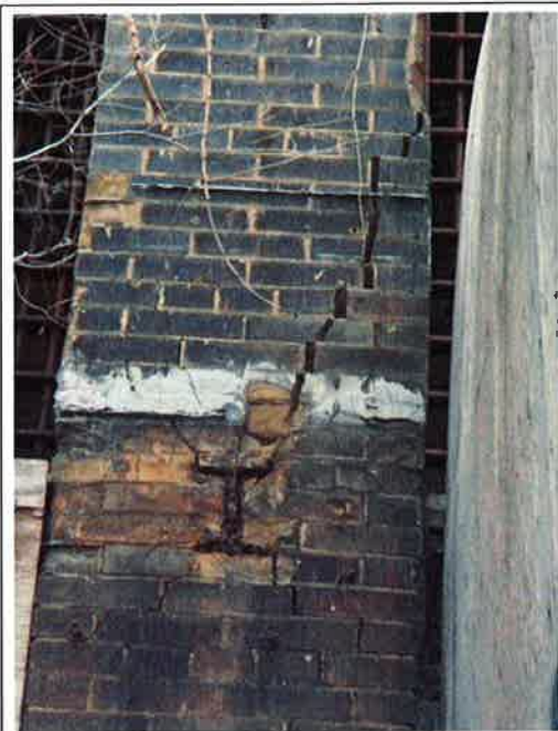
Photograph No. 8: Severe fracturing and displacement of the masonry column surrounding embedded steel beam (south façade) (CRITICAL CONDITION)
