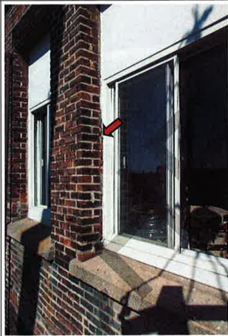
Photograph No. 29: Vertical crack along mortar filled joint at the masonry wall/window junction (south façade)
