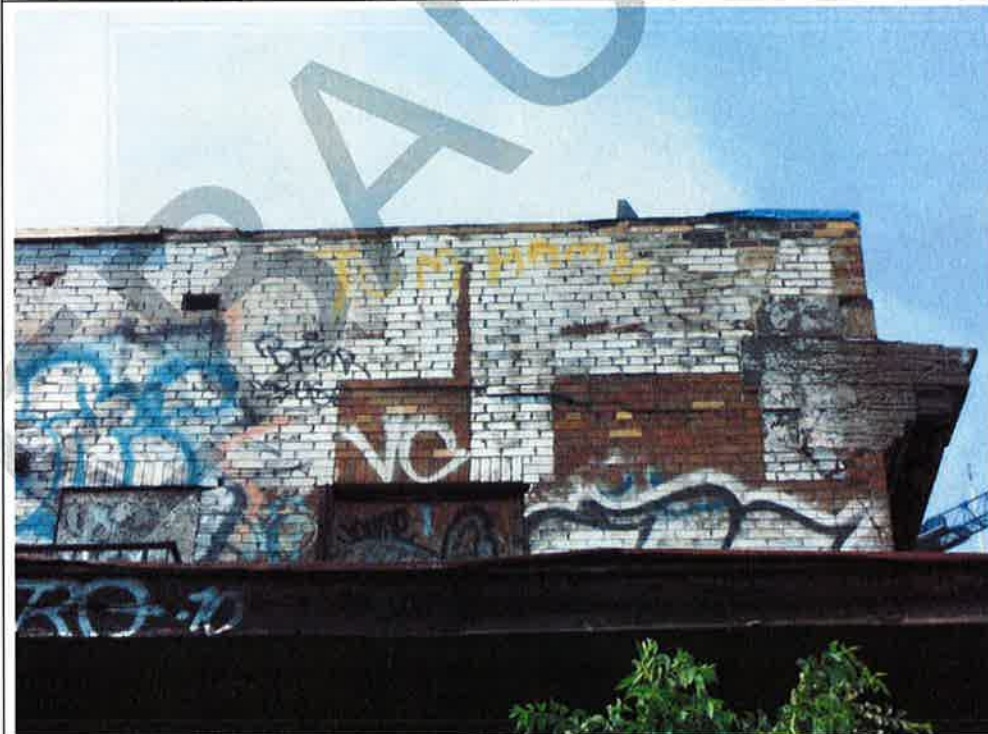
Photograph No. 10: Significant lateral displacement of the masonry elements at parapet level and displacement of the stone cornice (south façade) (CRITICAL CONDITION)
