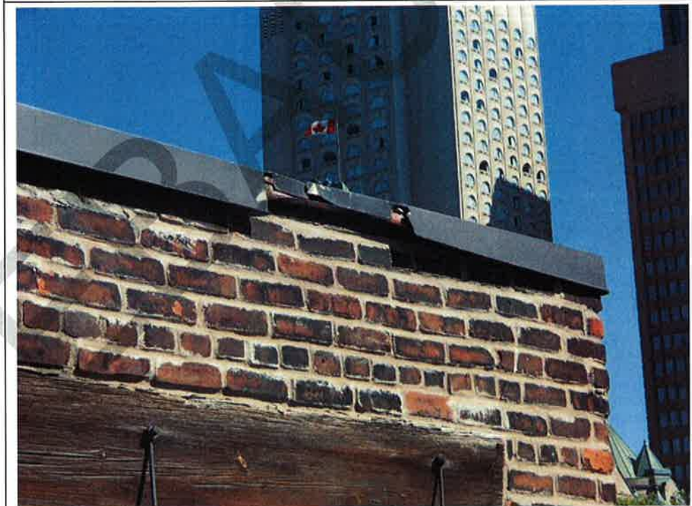
Photograph No. 43: Typical signs of localized damaged metal flashing (south façade)
