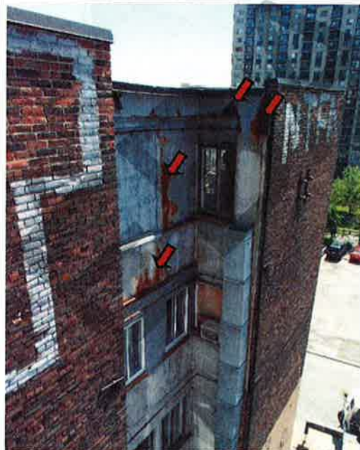
Photograph No. 40: Typical sign of heavily corroded, warped and poorly sealed metal sheet siding (west façade)
