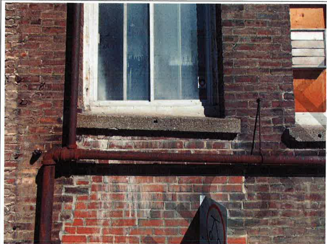
Photograph No. 39: Out of axis concrete window sill and localized step cracking of the mortar joints (south façade)
