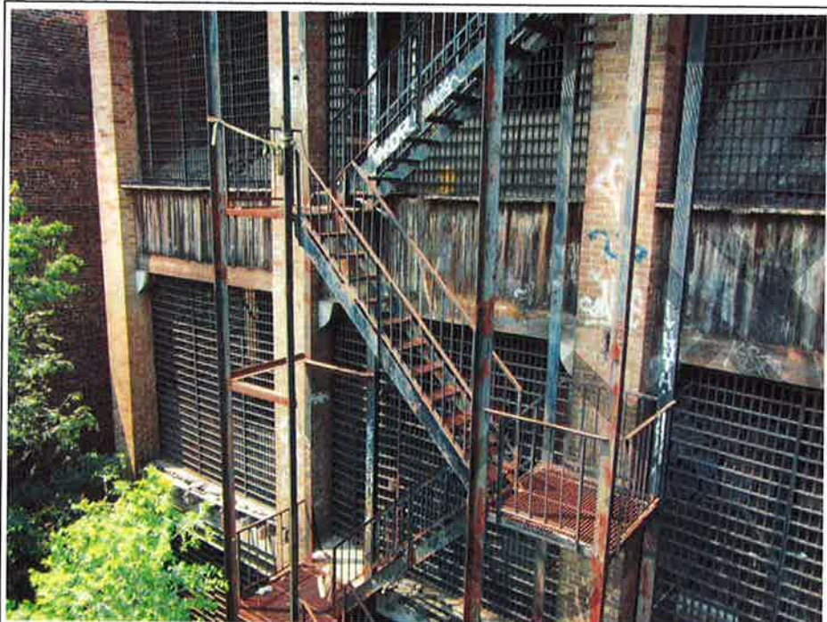
Photograph No. 59 : Building 1162 : General view of fire damaged balconies and fire escapes (south elevation)
