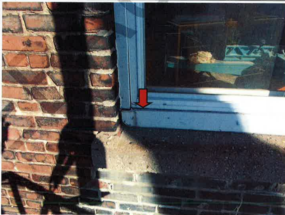
Photograph No. 84 : Building 1180: Damaged window frame (south elevation)
