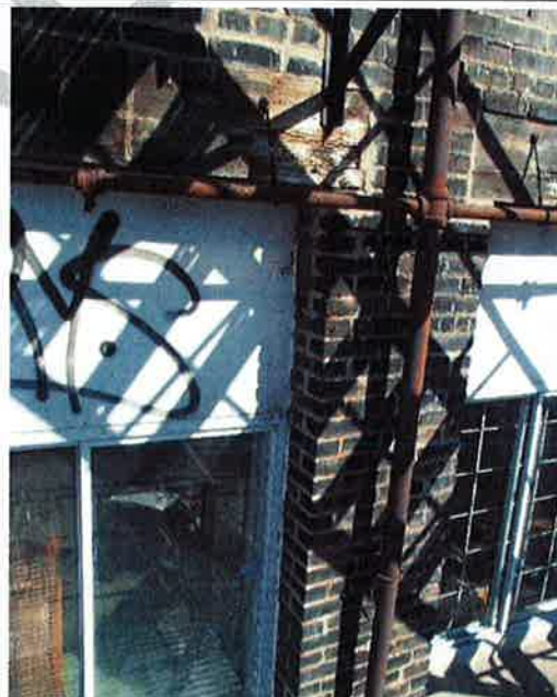
Photograph No. 41: Typical sign of external sprinkler network exhibiting widespread corrosion (south façade)
