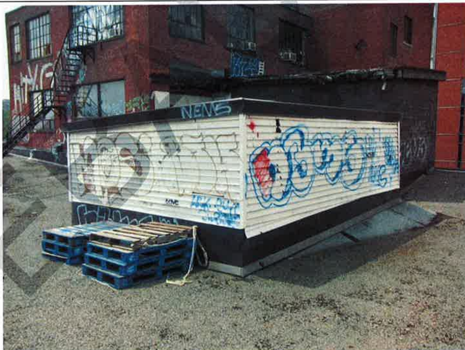
Photograph No. 78 : Building 1180: Typical patching of exterior walls ay penthouse (note the vinyl siding, sheet metal and plywood) (roof level)
