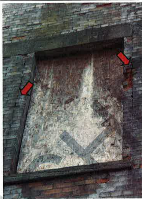
Photograph No. 9: Severe longitudinal cracking and spalling of the brick units (east façade) (CRITICAL CONDITION)
