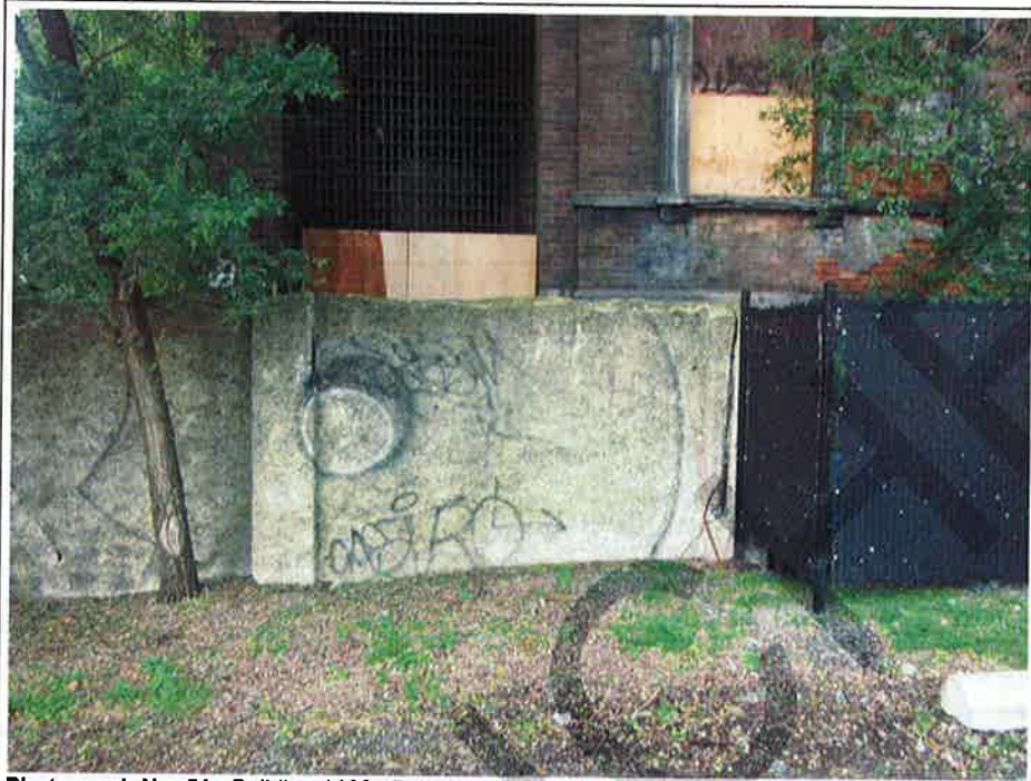
Photograph No. 51 : Building 1162 : Deterioration of the retaining wall (parking)
