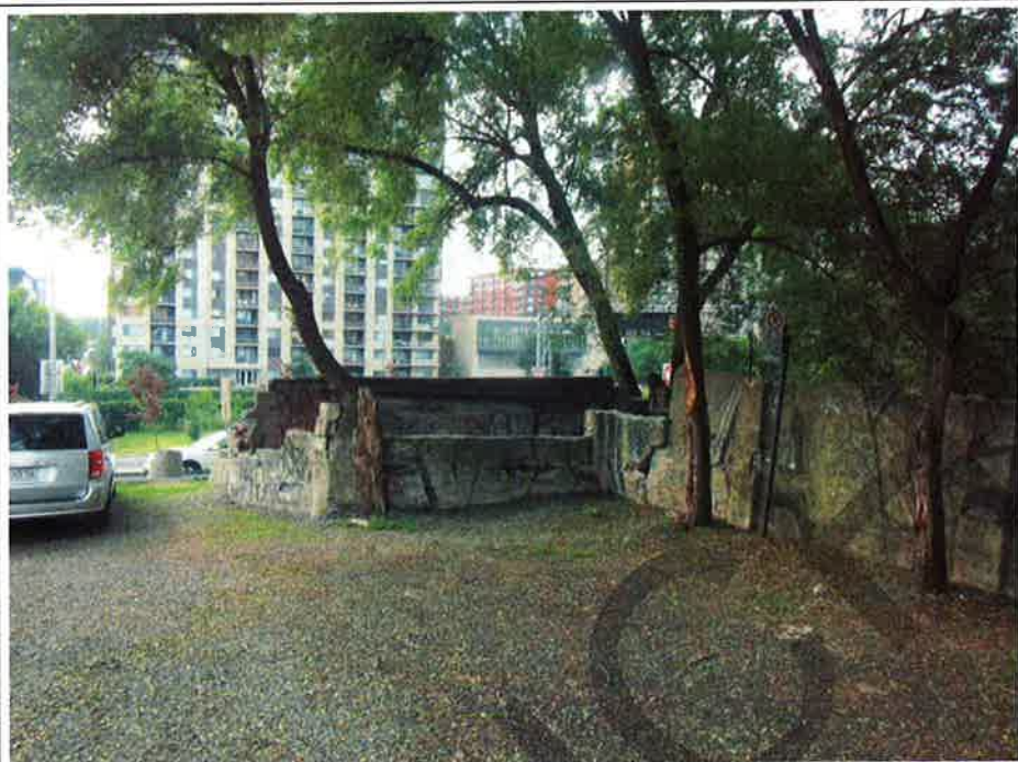
Photograph No. 53 : Building 1162 : Deterioration of the retaining wall (parking)
