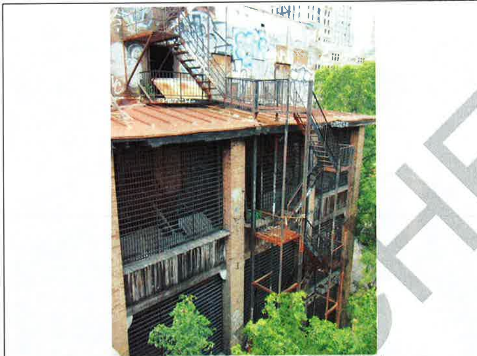
Photograph No. 57 : Building 1162 : General view of fire damaged balconies and fire escapes (south elevation)
