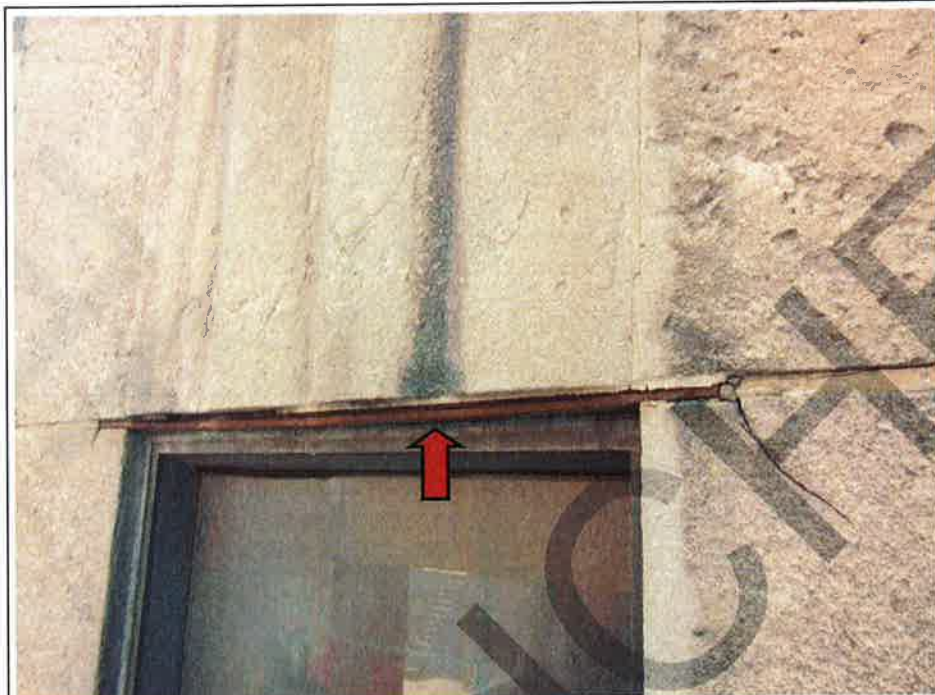
Photograph No. 69 : Building 1180 : Sagging steel lintel under stone panel (north elevation)
