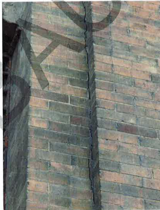
Photograph No. 50 : Building 1162 : Longitudinal cracking at brick offset (east elevation)
