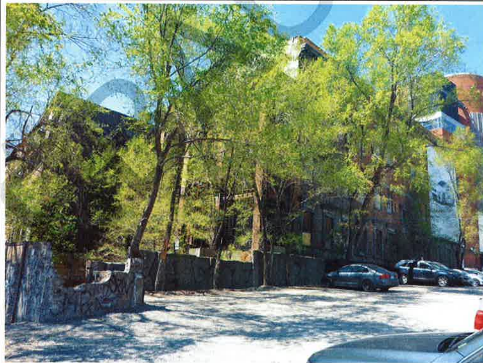
Photograph No. 12: Deteriorated concrete retaining wall along rear east façade
