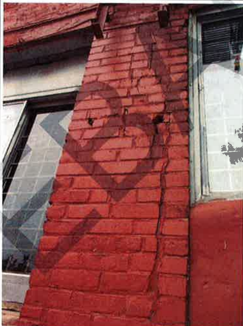
Photograph No. 22: Localized longitudinal cracking of masonry column cladding adjacent to window jambs (south façade) (CRITICAL CONDITION)
