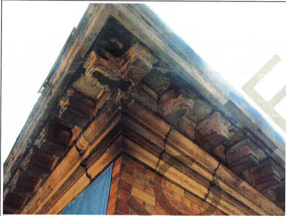
Photograph No. 55 : Building 1162 : Stone and dentil deterioration (northwest corner)
