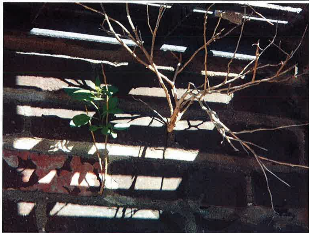
Photograph No. 31: Extreme vegetation growth between brick units (south façade)
