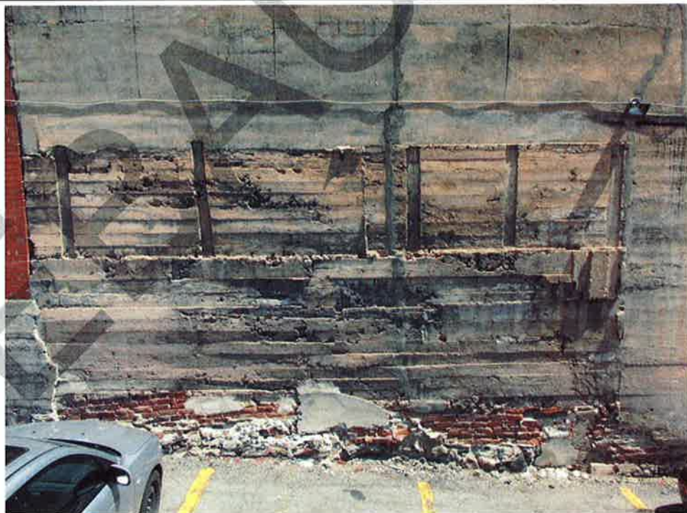
Photograph No. 34: Significant honeycombing and concrete delamination, and ongoing erosion of mortar, parging and brick (west façade)
