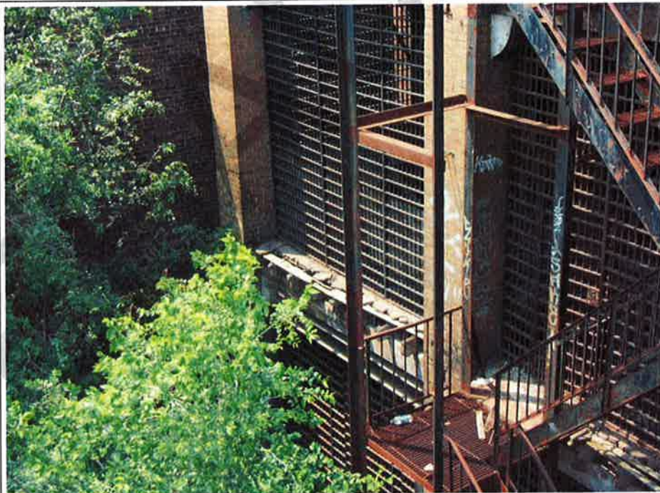
Photograph No. 58 : Building 1162 : General view of fire damaged balconies and fire escapes (south elevation)
