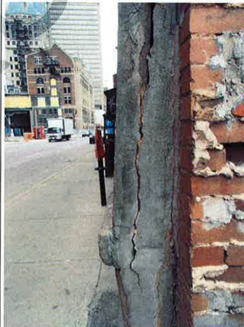
Photograph No. 23: Fracturing and lateral displacement of the stone cladding at the street level (north façade)
