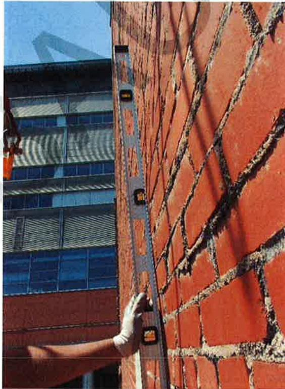
Photograph No. 27: Bowing/deflection of a portion of the brick masonry cladding (west façade)
