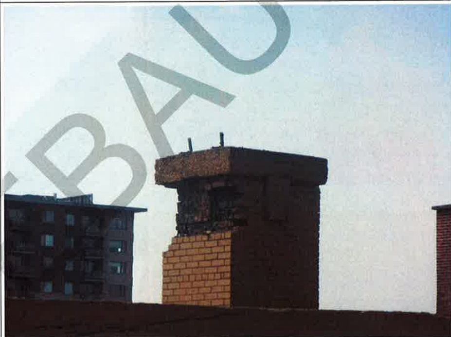
Photograph No. 54 : Building 1162 : Missing bricks (roof level)
