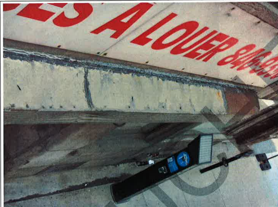
Photograph No. 73 : Building 1180 : Cohesive failure of caulking at metal flashing (north elevation)
