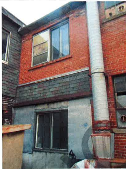
Photograph No. 77 : Building 1180: Typical patching of exterior walls (note the steel sheeting, asphalt shingles and bricks) (roof level)
