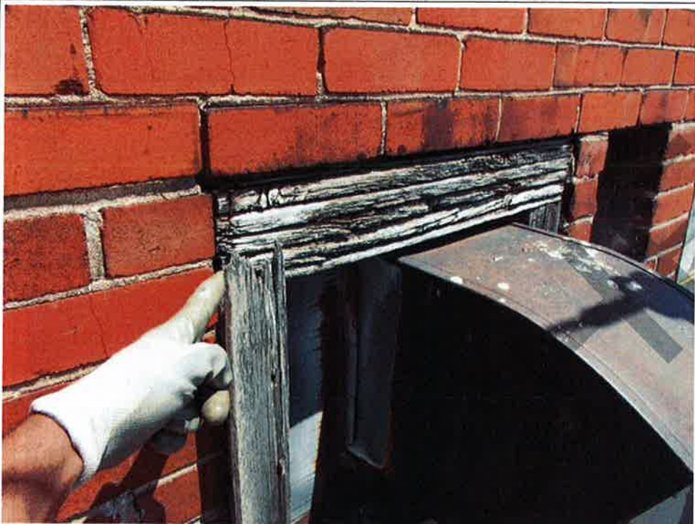
Photograph No. 44: Heavily deteriorated, rotted and splintered wood frame around exhaust duct (west façade)
