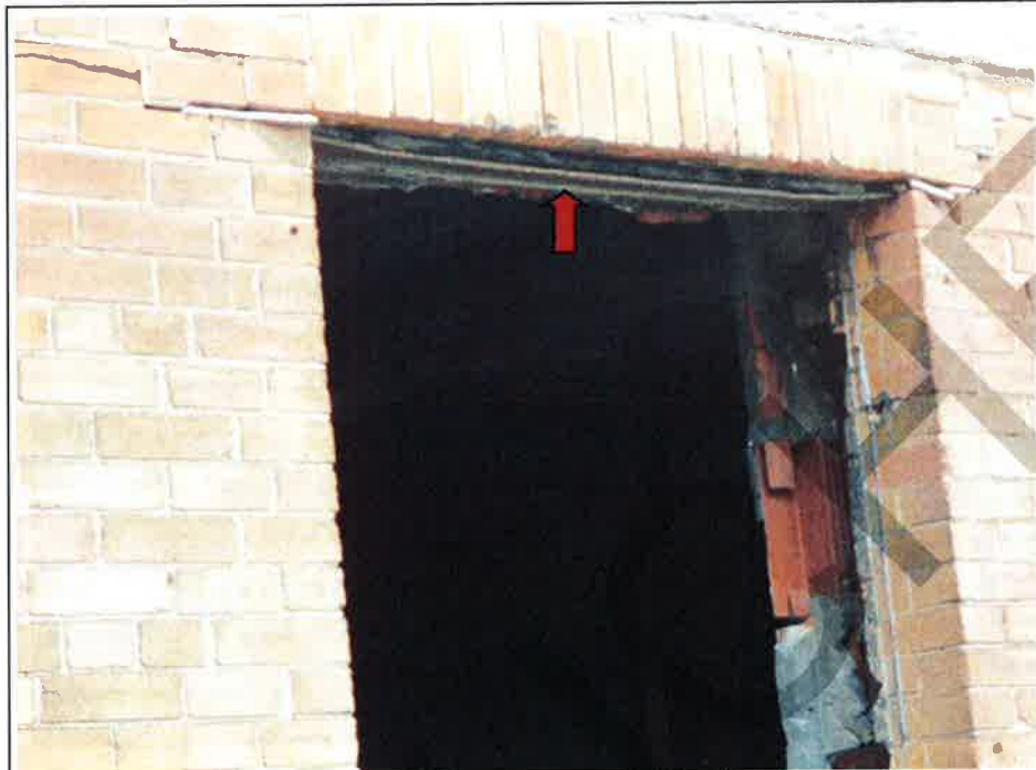
Photograph No. 61 : Building 1162 : Severe corrosion of steel lintel (west elevation)
