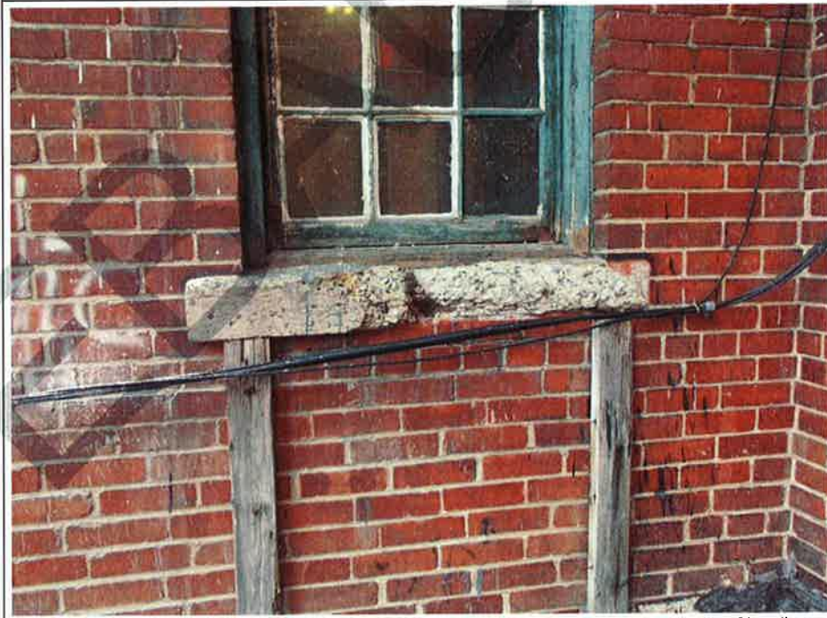
Photograph No. 82 : Building 1180 : Spalled concrete window sill (north elevation – roof level)
