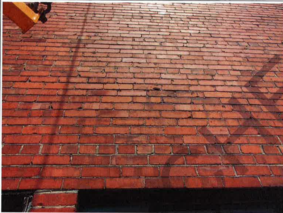
Photograph No. 26: Typical hairline cracking of the brick masonry units (west façade)
