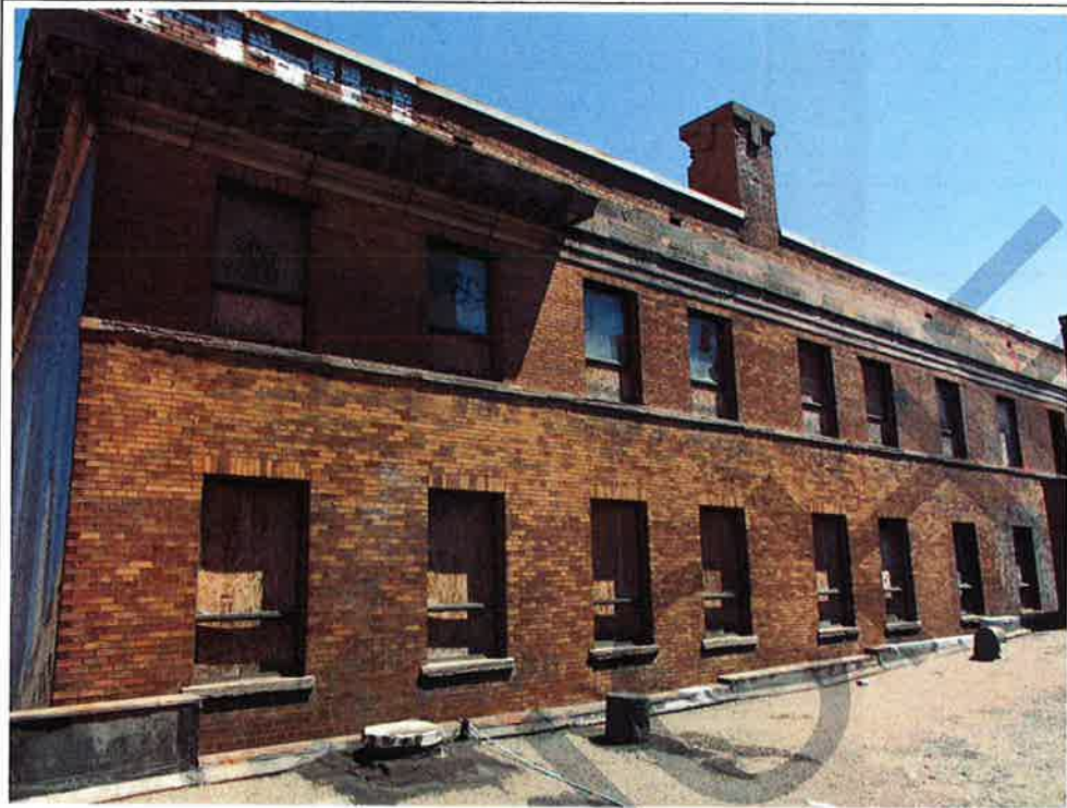
Photograph No. 16: Numerous missing window panes (west façade)
