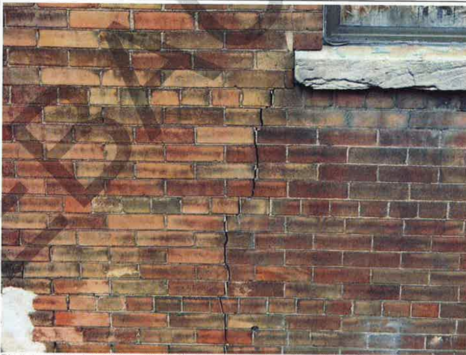
Photograph No. 60 : Building 1162 : Typical longitudinal cracking of bricks (west elevation)
