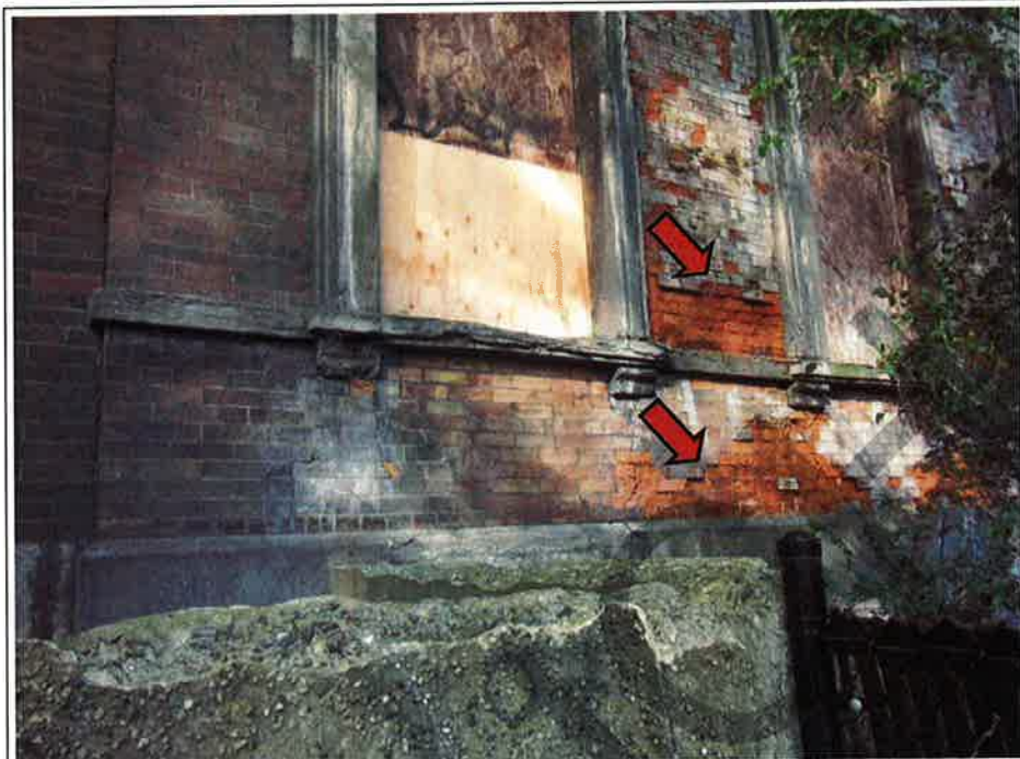
Photograph No. 49 : Building 1162 : Severe spalling of bricks (east elevation)
