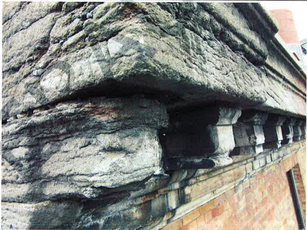
Photograph No. 17: Mortar erosion and significant flaking and erosion of ornamental stone dentil at cornice level (southeast corner)
