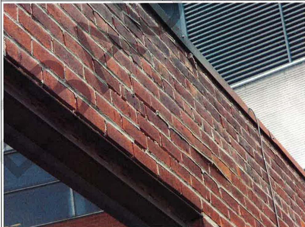
Photograph No. 30: Poorly bonded and spalled mortar joints (east façade – roof level)
