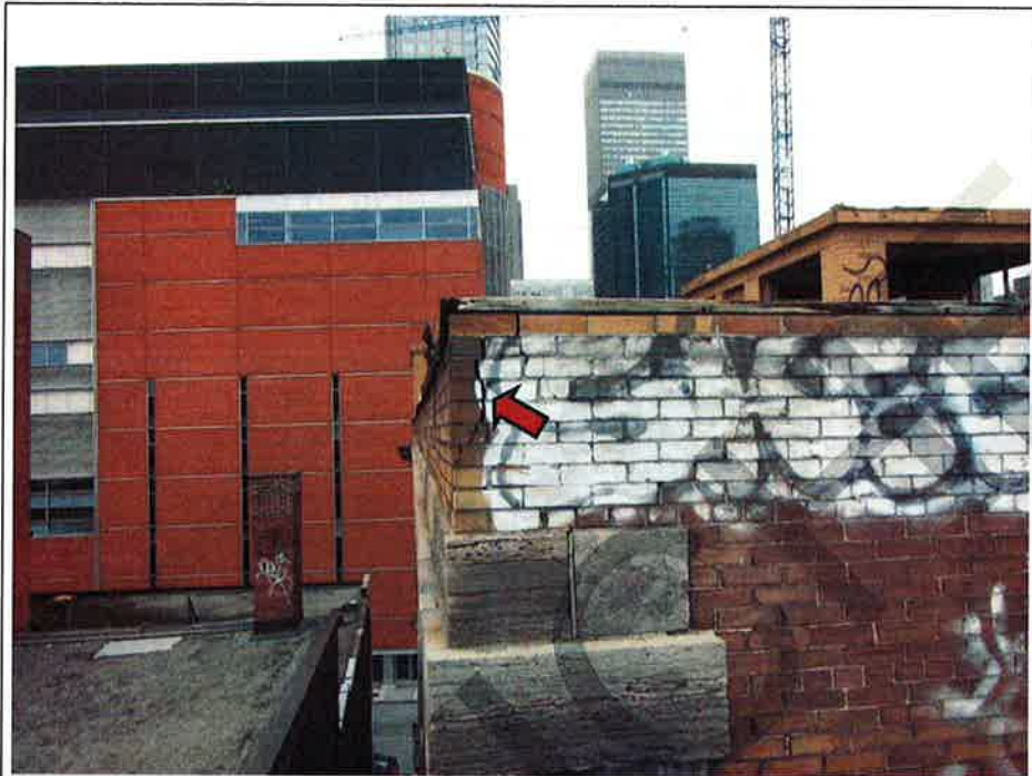
Photograph No. 67 : Building 1162 : Cracked masonry (southwest corner)
