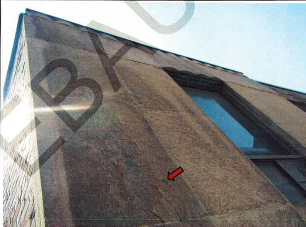
Photograph No. 32: Typical flaking of cut stone surface (north façade)
