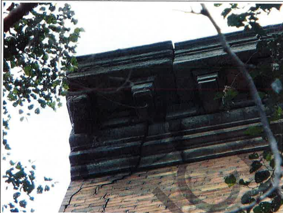
Photograph No. 11: Displacement and severe fracturing of the brick masonry, stone cornice and dentils (southeast corner) (CRITICAL CONDITION)
