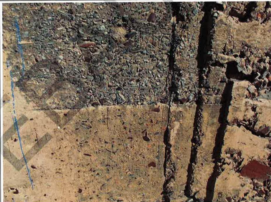
Photograph No. 86 : Building 1180: Typical aggregate settlement and honeycombing of concrete wall (south elevation)
