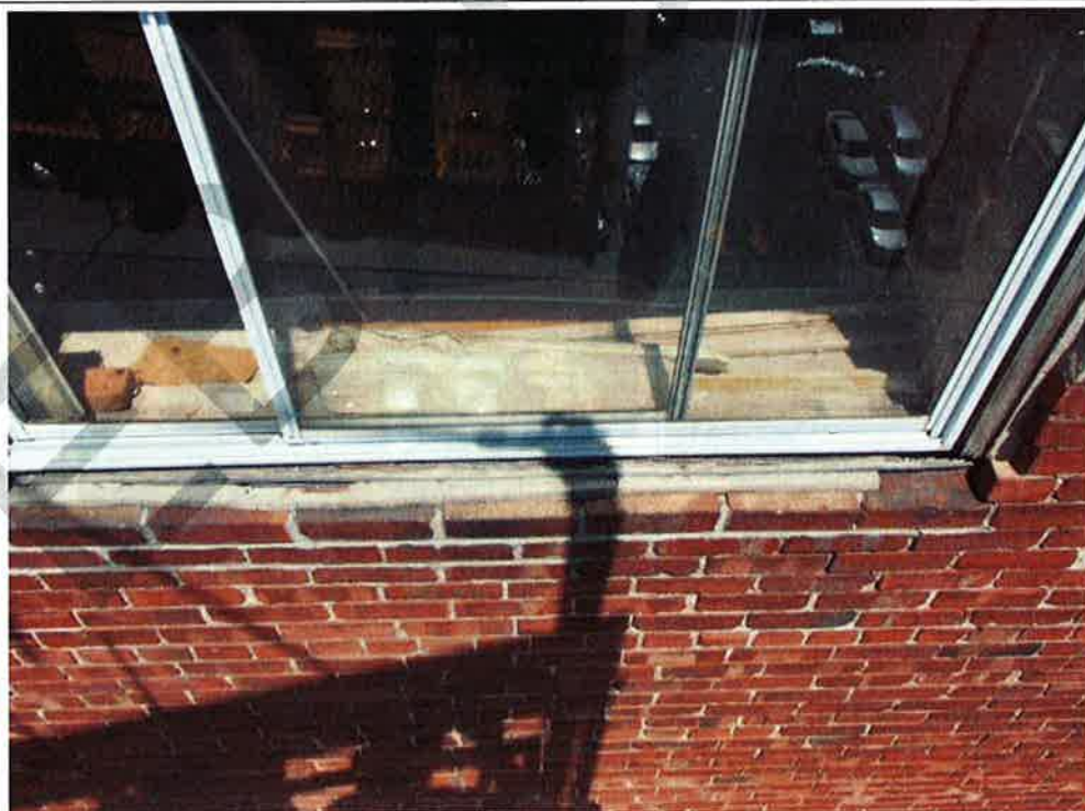
Photograph No. 38: Typical sign of missing window sill or metal flashing (west façade)
