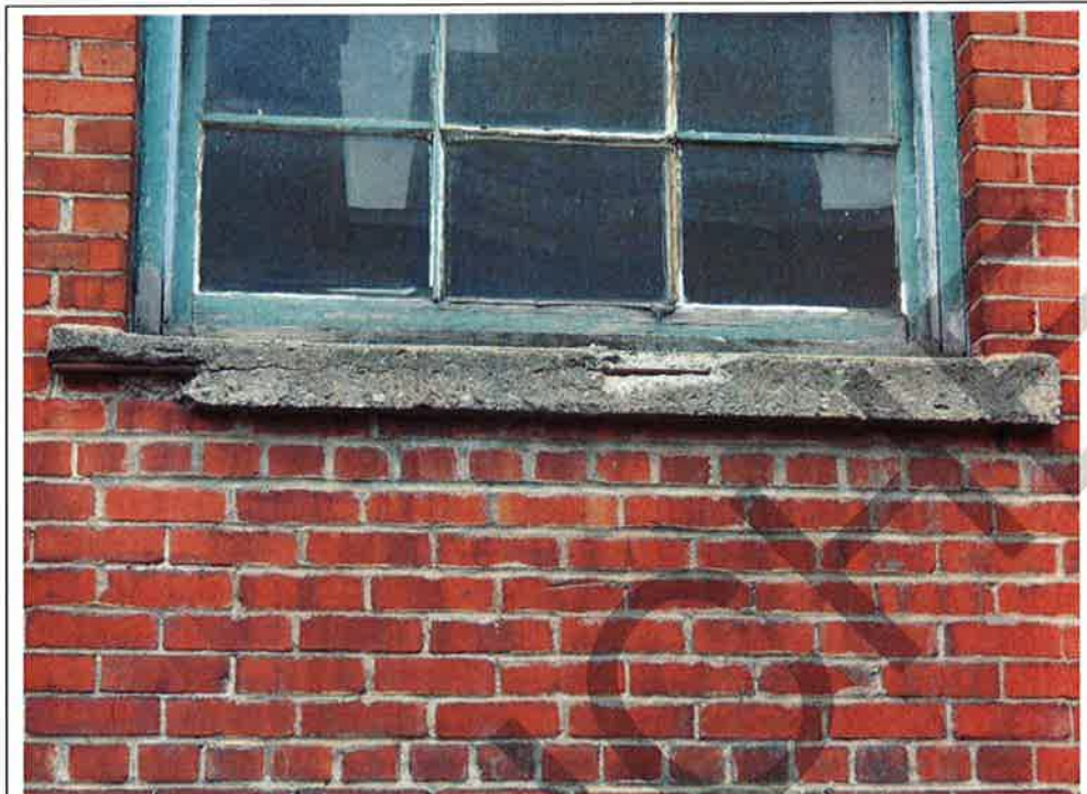
Photograph No. 33: Fractured concrete window sill with exposed and corroded steel reinforcement (east façade – roof level)
