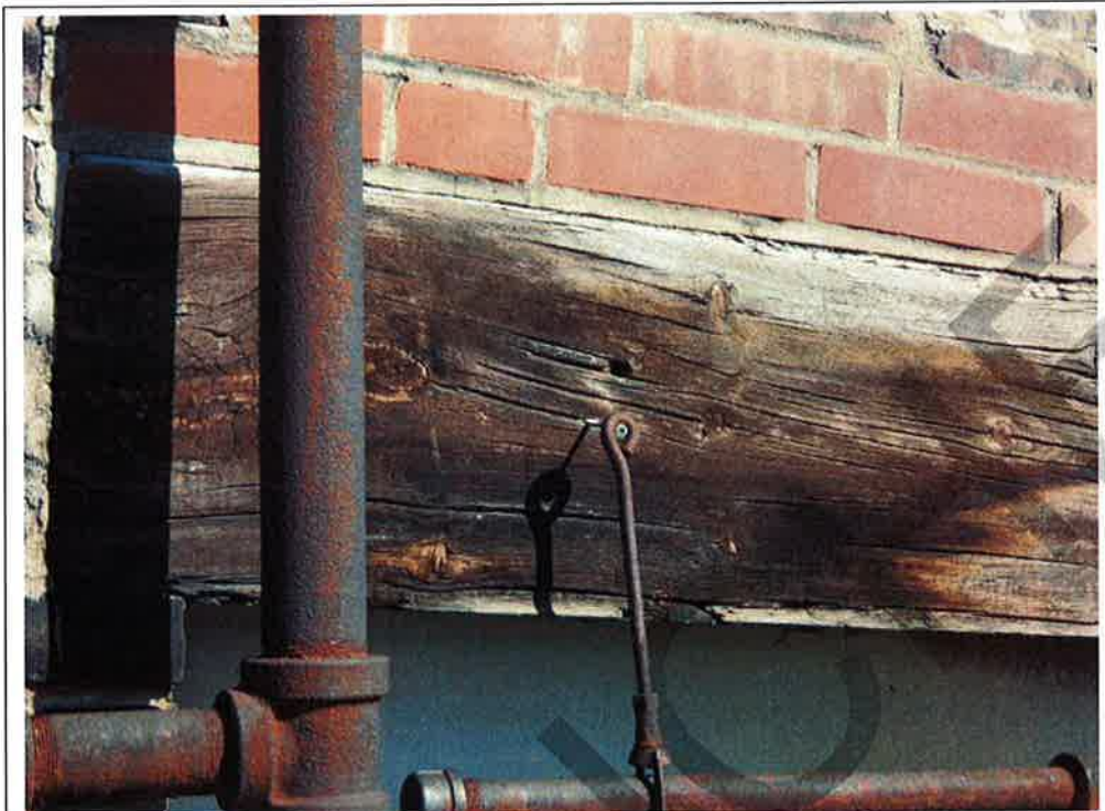
Photograph No. 42: Typical signs of inadequate anchoring of the sprinkler pipe (south façade)
