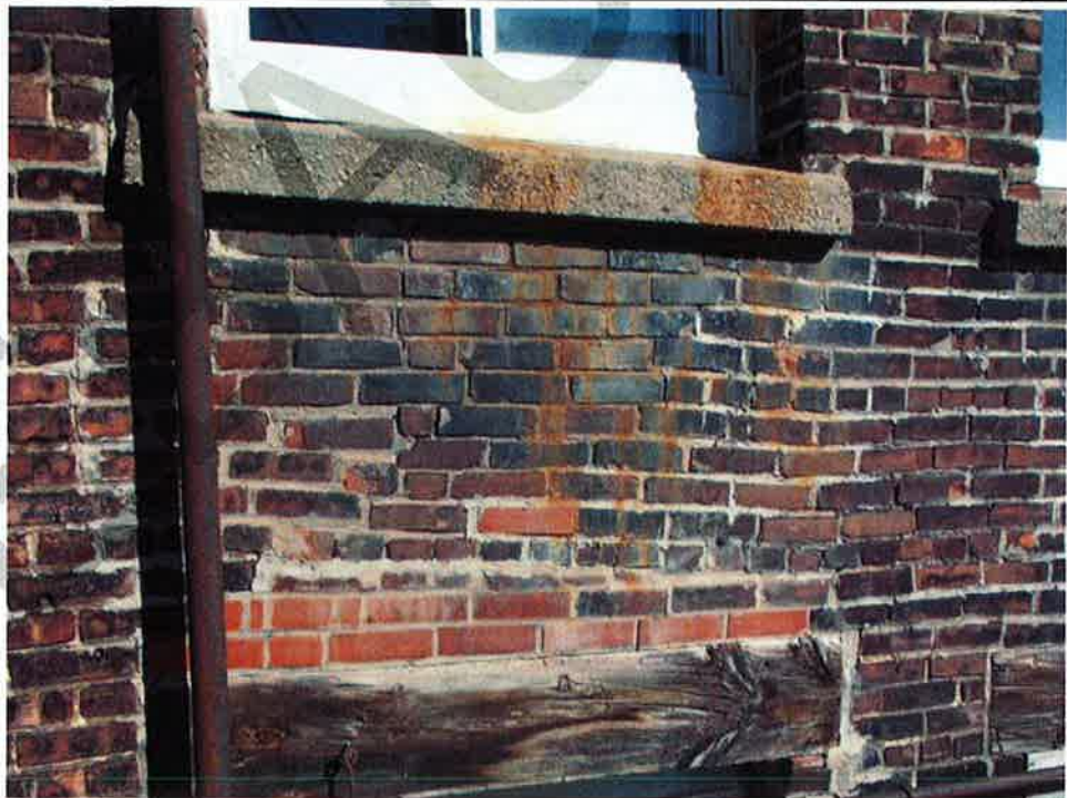
Photograph No. 36: Rust staining on and below concrete window sill. Note significant misalignment of window base and brick courses (south façade)
