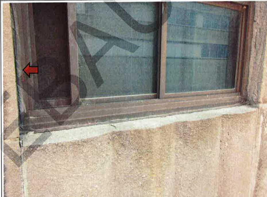
Photograph No. 70 : Building 1180 : Cohesive failure of caulking (north elevation)
