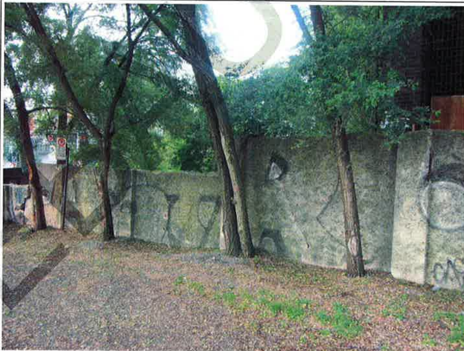
Photograph No. 52 : Building 1162 : Deterioration of the retaining wall (parking)
