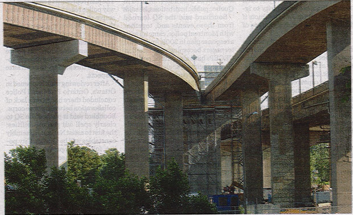
Crews are beginning the process of rebuilding what’s called the Montreal West interchange, and Transport Quebec says it will take until 2020 for the work to be completed. MARIE-FRANCE COALLIER/MONTREAL GAZETTE FILES
