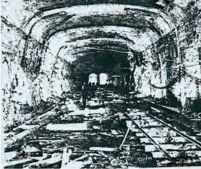
Construction du tunnel ferrovière, c. 1913, tiré de Anthony Clegg (2008), The Mount Royal Tunnel. Canada's First Subway , Pickering, Railfare DC Books.
