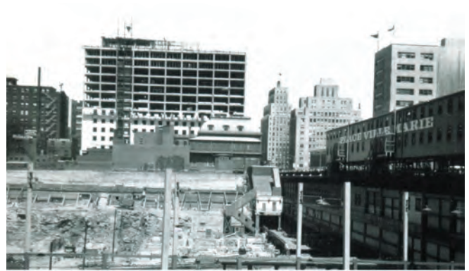
Vue de la construction de la Place Ville Marie, tiré de Anthony Clegg (2008), The Mount Royal Tunnel. Canada's First Subway , Pickering, Raifare DC Books.
