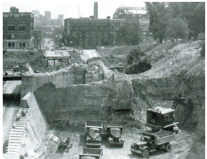
Angle des rues Mansfield et De LaGauchetière, c. 1952, tiré de Anthony Clegg (2008), The Mount Royal Tunnel. Canada's First Subway , Pickering, Railfare DC Books.
